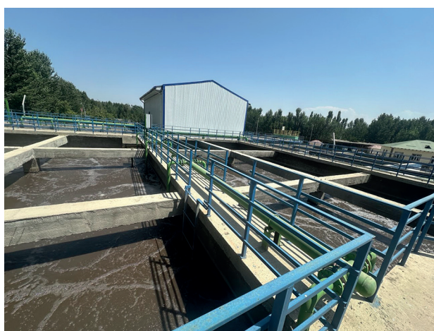
Sewage facility in Markhamat district of Andijan region
